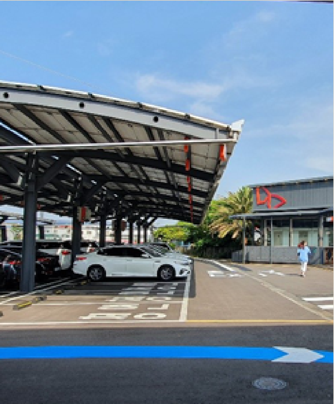
Solar-panel carport, SK Rent-a-Car Jeju branch
